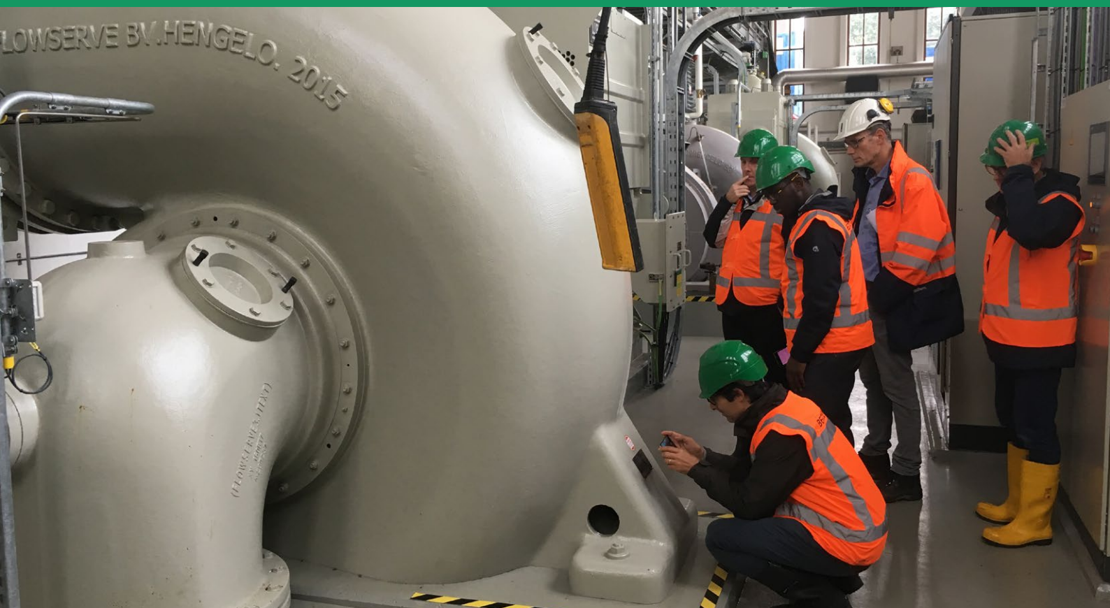
Pumping station at Eefde, NL
