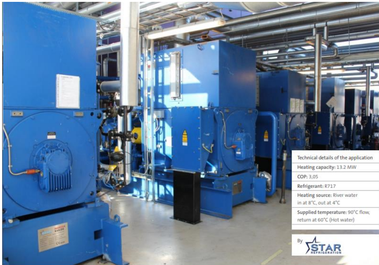
Figure 15: Heat pumps in Drammen district heating [19]
