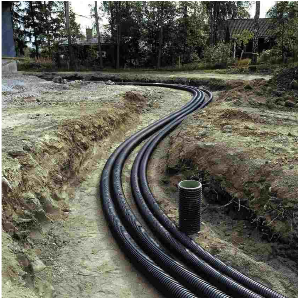
Figure 32: Flexible 4DHC distribution pipes [26]
