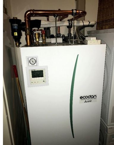
Heat pump connected to EMS
