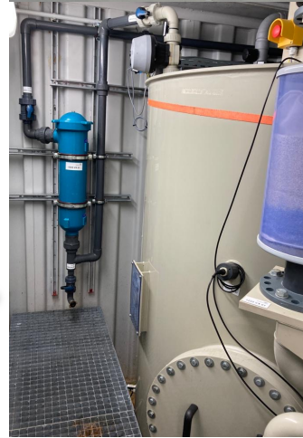
4 m 3 Mixing tank (homogenization)
