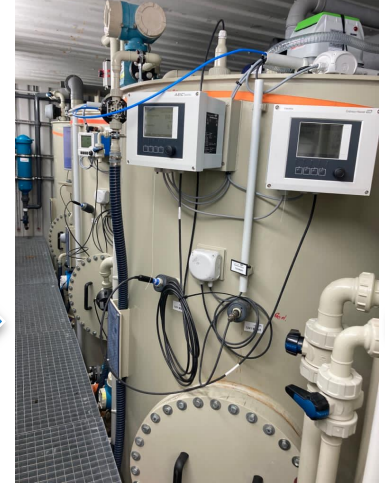
4 m 3 Reactor 2 (micro-aerobic, biomass growth)
