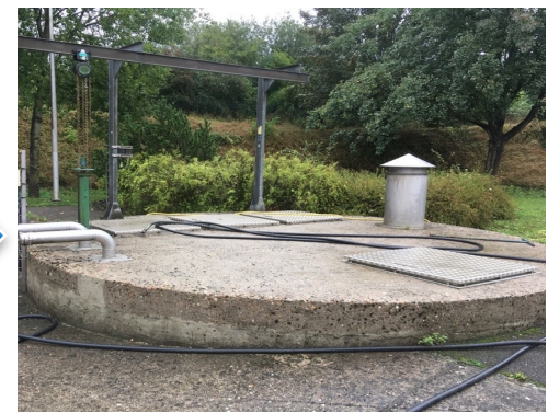
Storage tank (effluent)
