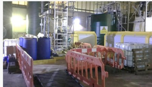
Peel Common WWTP, UK Southern Water
