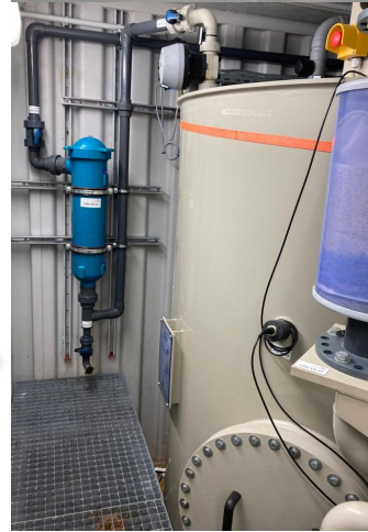
4 m 3 Mixing tank (homogenization)
