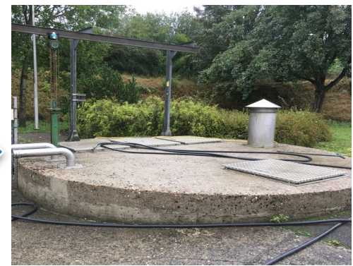
Storage tank (effluent)
