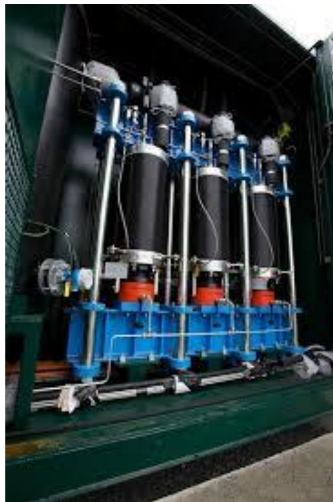
ITM Power stacks in 2017 plant
