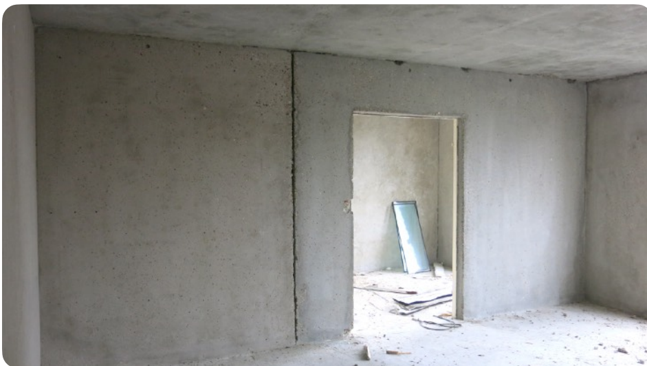
Prefabricated walls after stripping of interior linings and removal of asbestos from surfaces, before demolition or deconstruction of the building.
