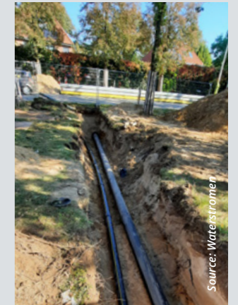
Separate piping was installed between the paper mill and the waste water treatment plant.
