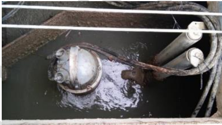
Figure 1 – Seend PS wet well showing Pump 2
