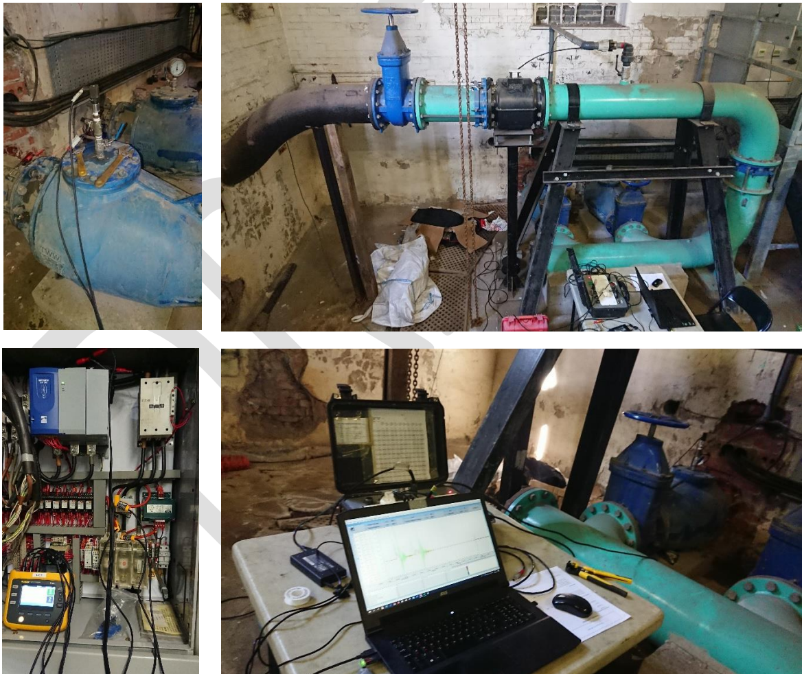
Figure 1 – Photographs taken during site audit (Top left: pressure transducer connected to top of check valve, Top right: Common discharge pipework and flow meter arrangement, Bottom left: 'Fluke' meter connected to terminals inside MCC; Bottom right: Data recorder and laptop)
