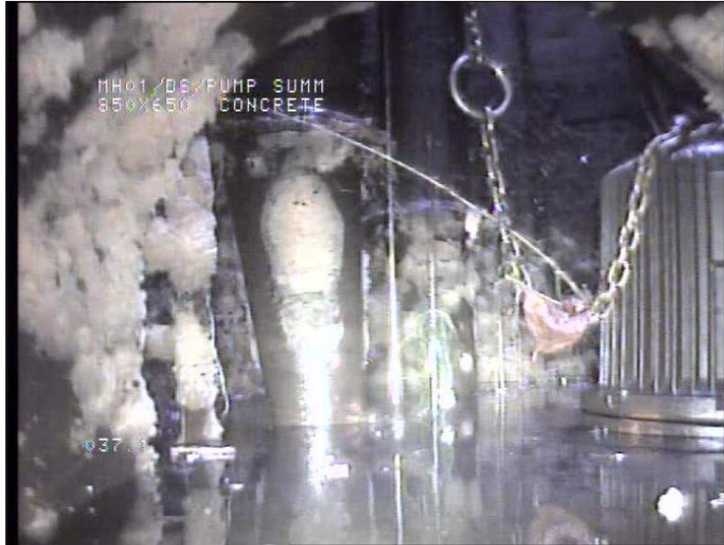
Photo: 2_15a 37.2m, General Observation, Remark: Pumps at Pump Sump Chamber
