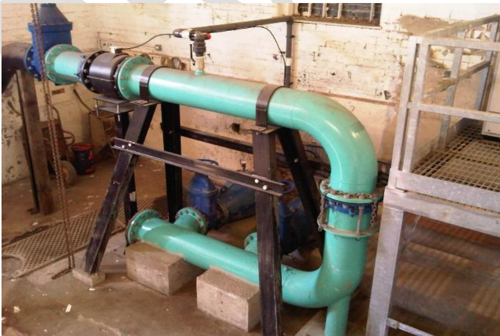
Figure 4 – Tinsley Pump Station basement area pipework
