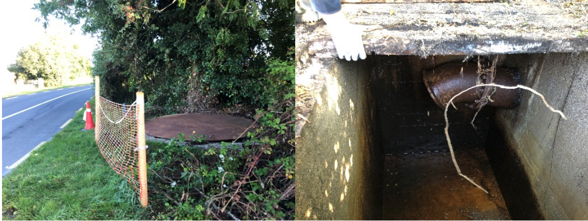
Figure no. 19: Lock 16 PS Outfall
