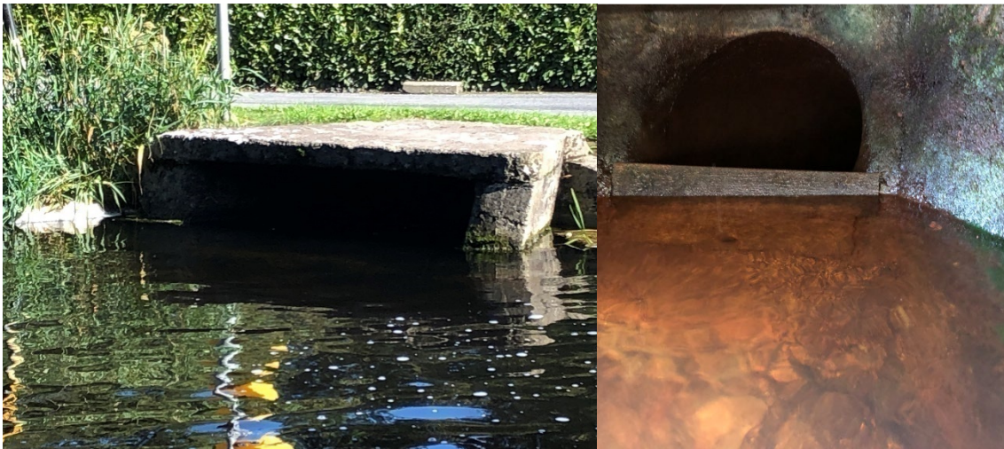
Figure no. 20: Lock 17 PS Outfall
