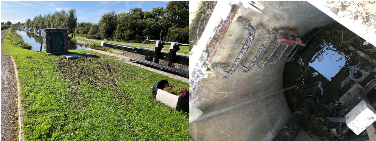
Figure no. 27: Lock 35 PS on the Grand Canal (Left); Inside Lock 35 PS wet well (Right)
