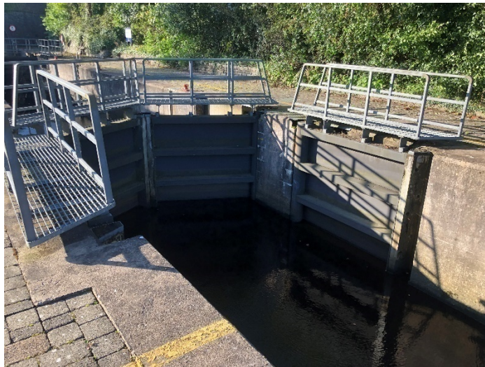
Figure no. 39: Drumshanbo Dual Lock Station
