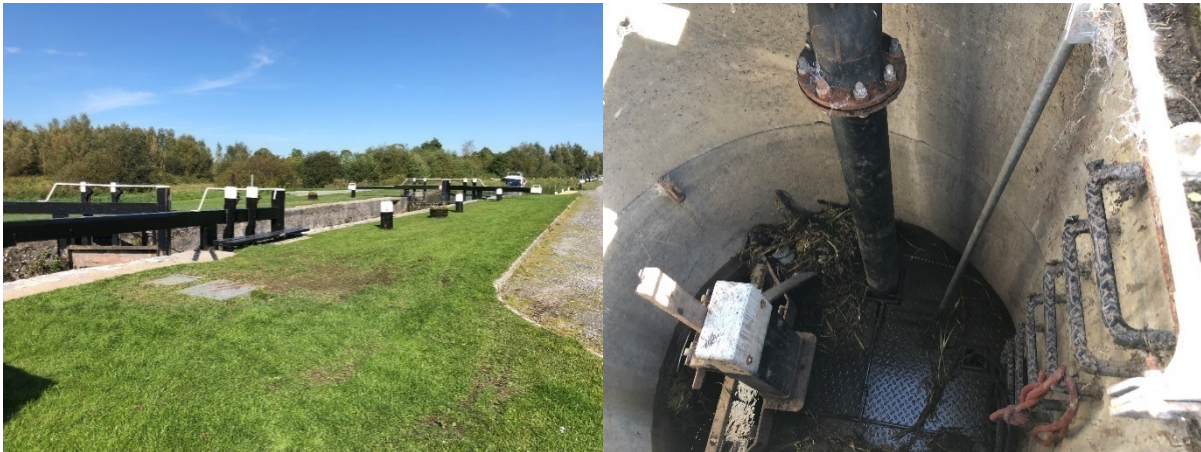
Figure no. 26: Lock 36 PS on the Grand Canal (Left); Inside Lock 36 PS wet well (Right)
