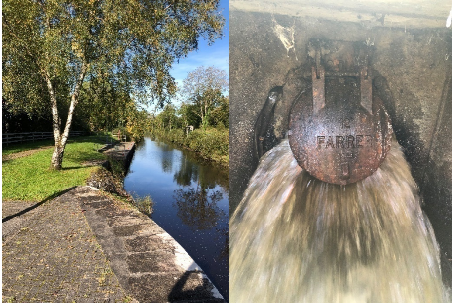
Figure no. 37: Drumleague PS Outfall viewed from the Lock (left); Rising Main outfall Farrer 12" flap valve on outlet (Right)
