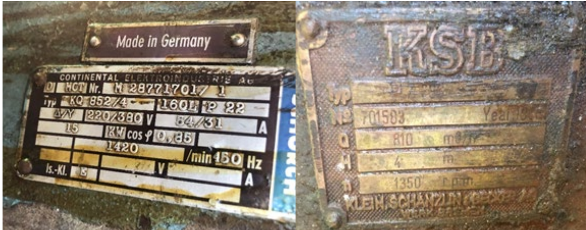
Figure no. 34: Richmond Harbour Existing Pump Nameplates
