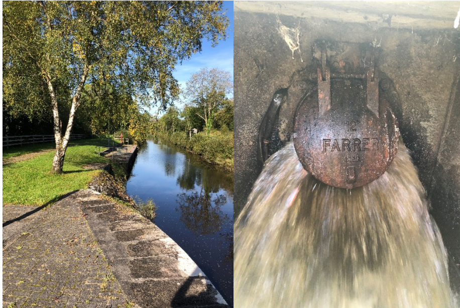
Figure 2 - Drumleague PS Outfall viewed from the Lock (left); Rising Main outfall Farrer 12" flap valve on outlet (right)
