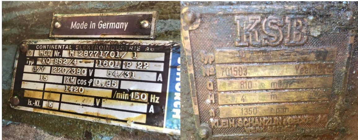
Figure 2 Richmond Harbour Existing Pump Name plates
