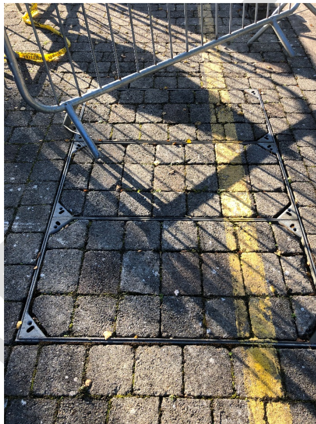
Figure 2 -Drumshanbo PS Wet well- Concrete top covers
