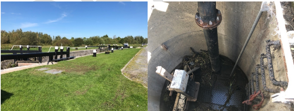
Figure 1 - Lock 36 PS on the Grand Canal ( Left); Inside Lock 36 wet well (right)
