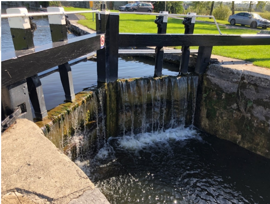
Figure 9 – Over topping of lock gate at Lock 35
