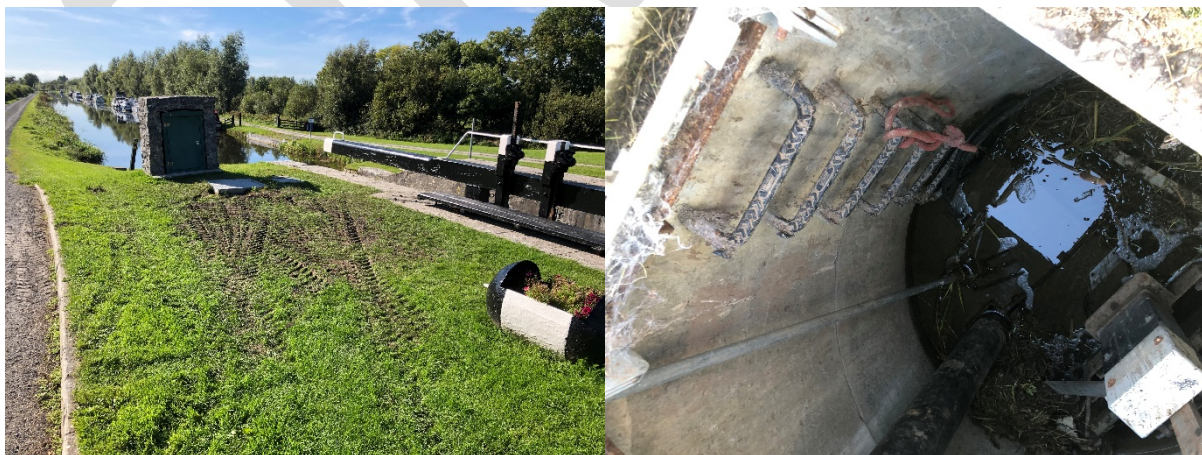
Figure 5 - Lock 35 PS on the Grand Canal ( Left); Inside Lock 35 wet well (right)
