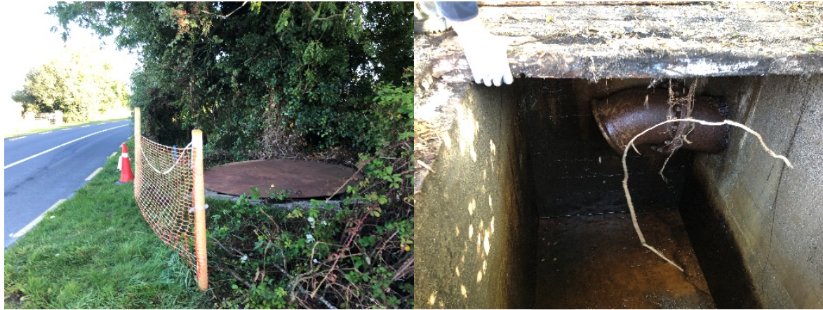
Figure 2 Lock 16 PS Outfall
