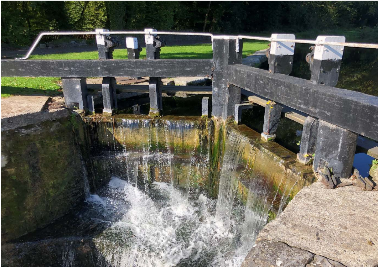
Figure 14 – Over topping of lock gate at Lock 17
