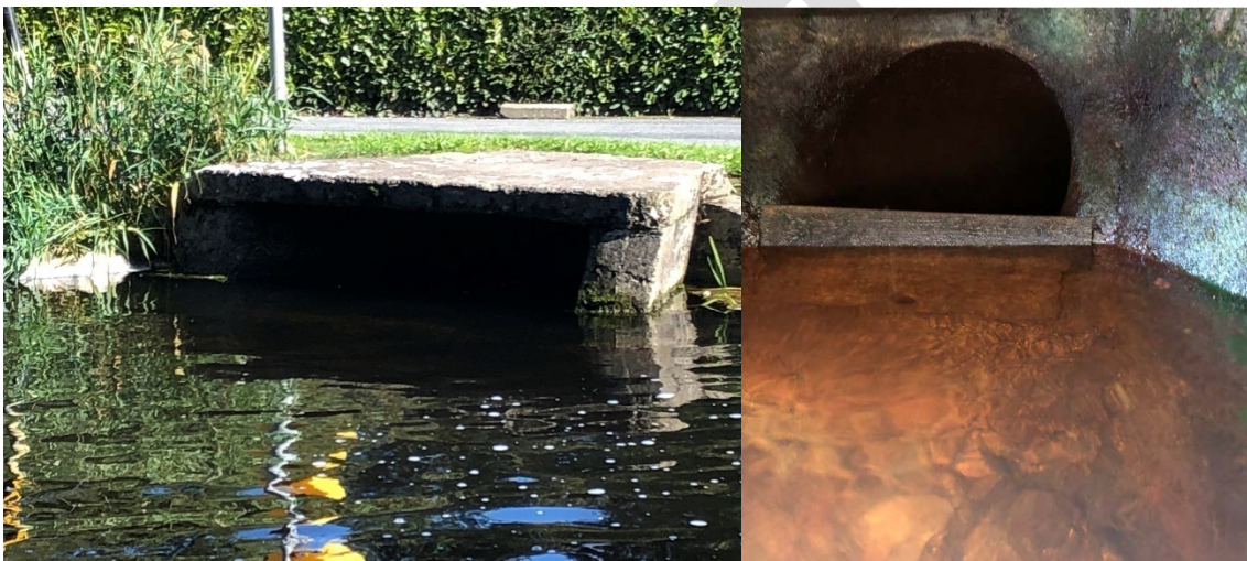
Figure 6 Lock 17 PS Outfall
