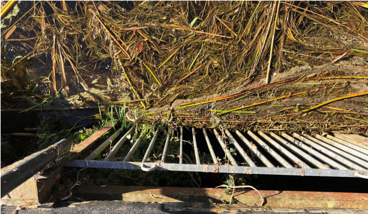
Figure 13 – Debris build up on the intake screen of Lock 18
