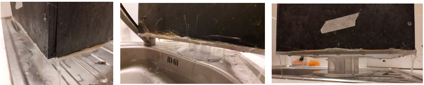
Leakage of the water
