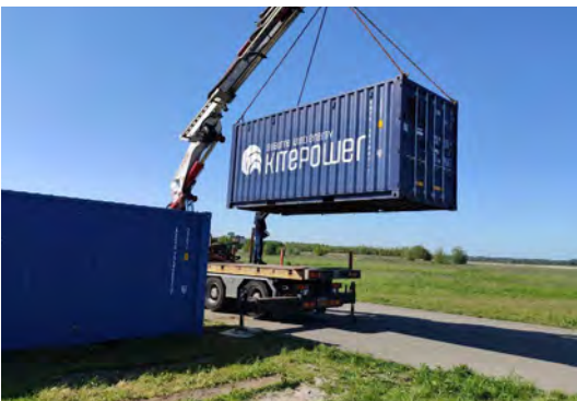
Figure 5 Containerised ground base station (Source: Kitepower)
