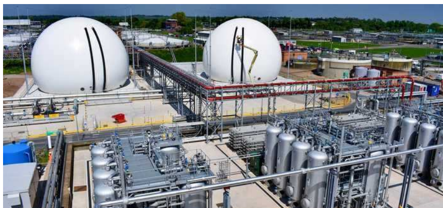
Figure 8-7: Minworth Sludge treatment plant. Showing the new THP plant in the foreground and the gas bags and MAD plant in the background
