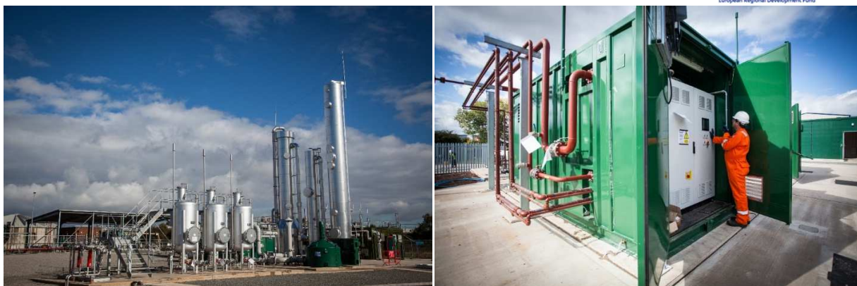
Figure 8-9: Biomethane Upgrading plant at Minworth (left) and Wartsila Gas compression unit (right)
