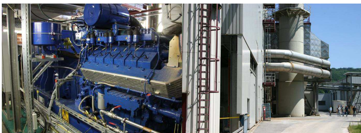
Figure 3-3: Combined heat and power unit and sludge incineration plant at WWTP Buchenhofen, Germany
