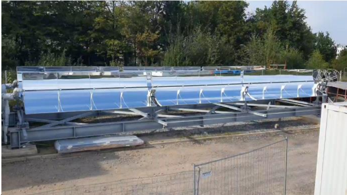
FIGURE 5. CSP installed in Bochum.
