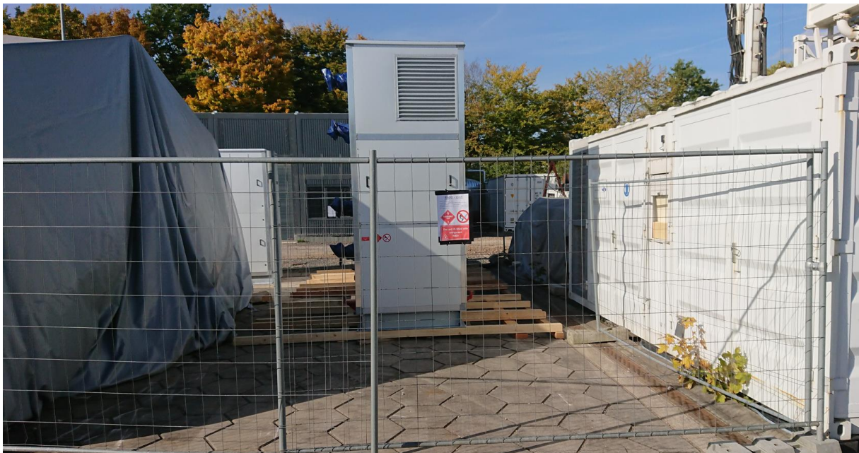
Figure 8. Ex-Zone Butane unit at Fraunhofer IEG
