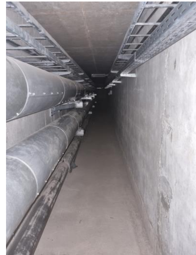
Figure 14.c. Insulated piping in DH tunnel
