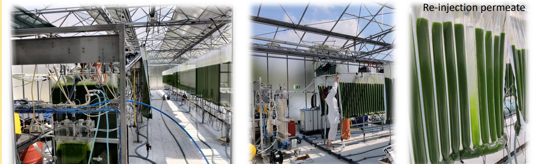
Figure 6: MAF connected to photobioreactor in Jülich (Germany).
