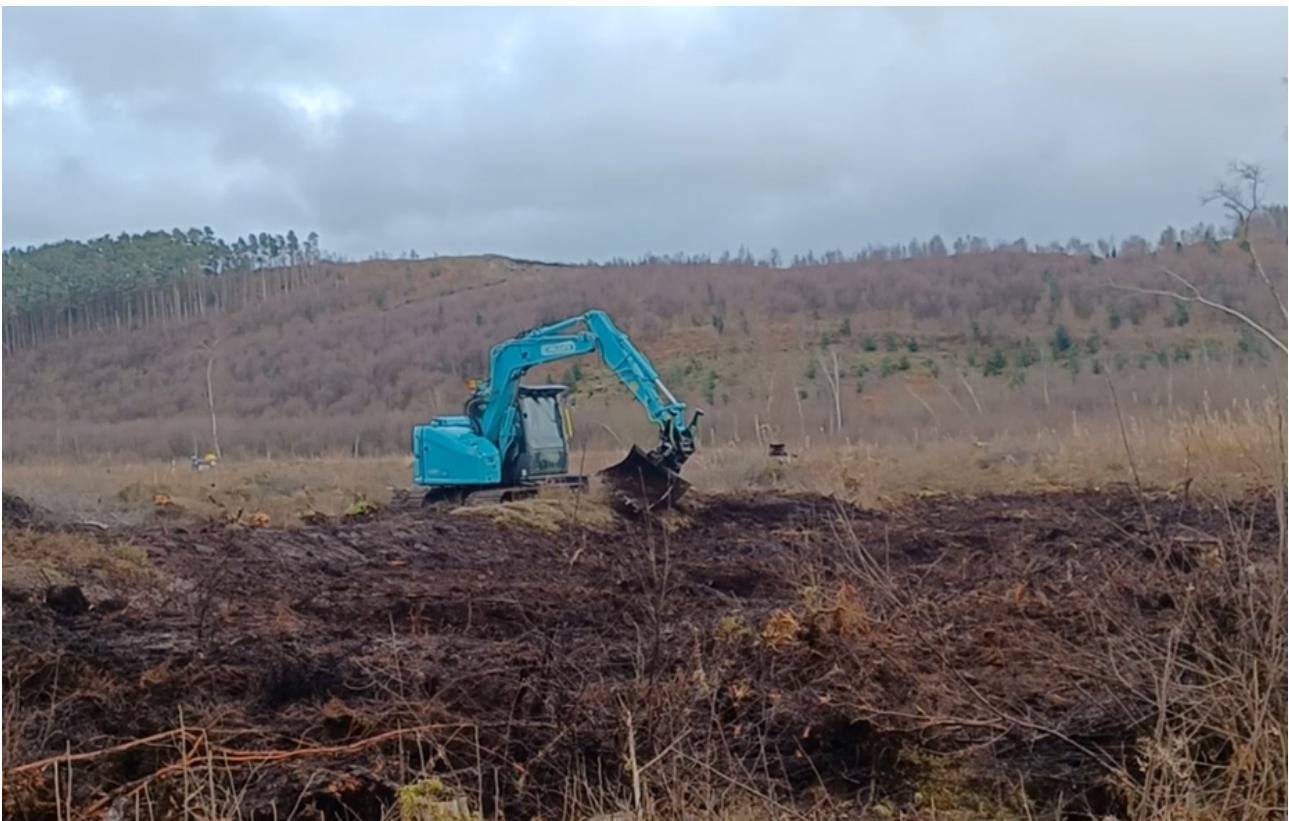
Figure 2.3: Excavator creating a section of bund, using a tilt-and-rotate coupler to increase the freedom of movement of the excavator bucket.
