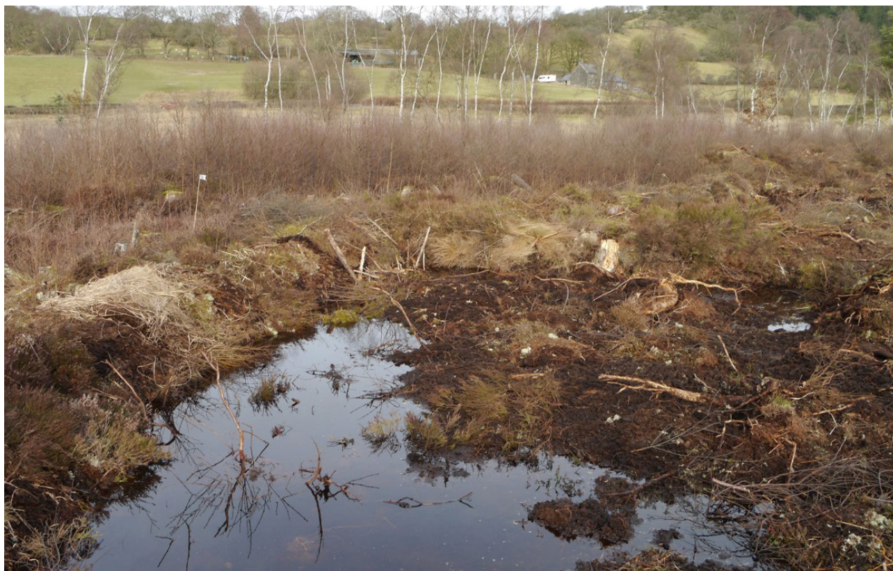
Figure 2.4: Newly completed bund, recovered with vegetation. The borrow pit created to source good quality peat for the bund is in the foreground, and has already started to fill with groundwater.
