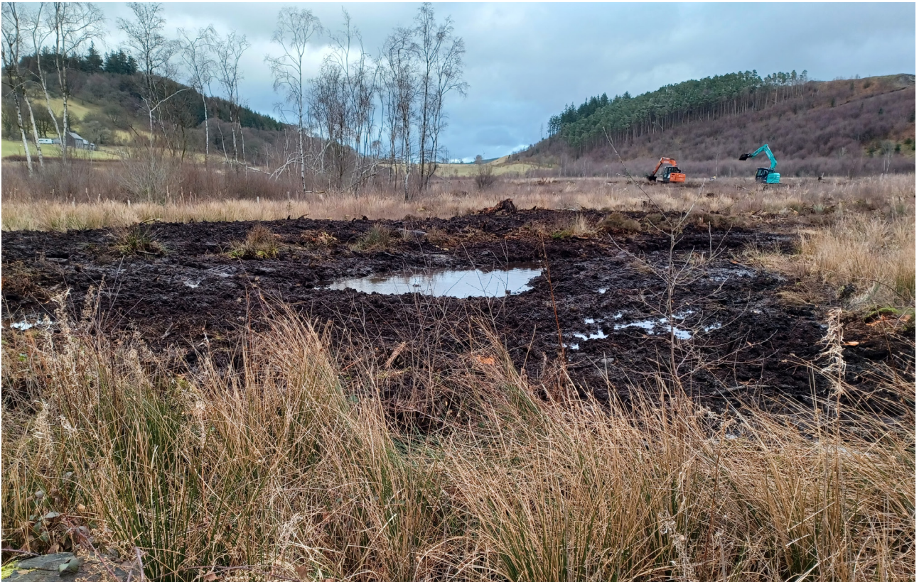
Figure 2.6: Newly completed pond, the deeper central section (partially filled with groundwater) is surrounded by a wide scrape.
