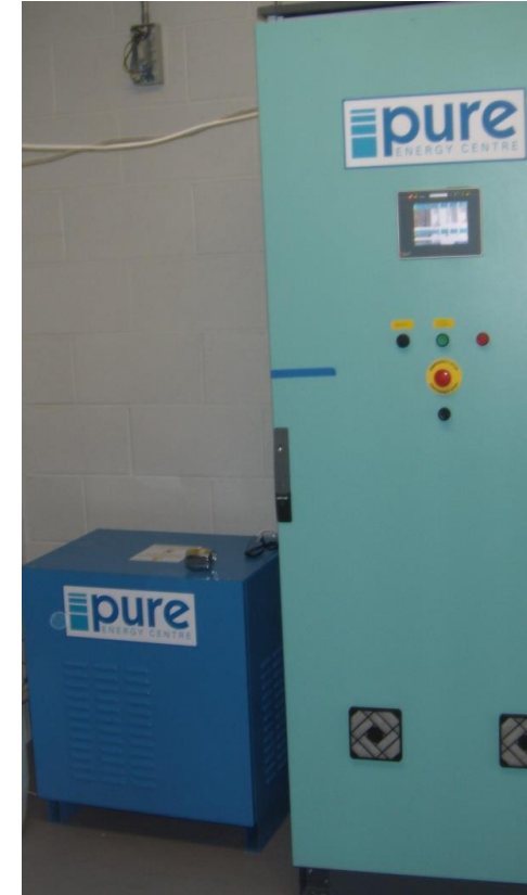
The electrolyser control system
