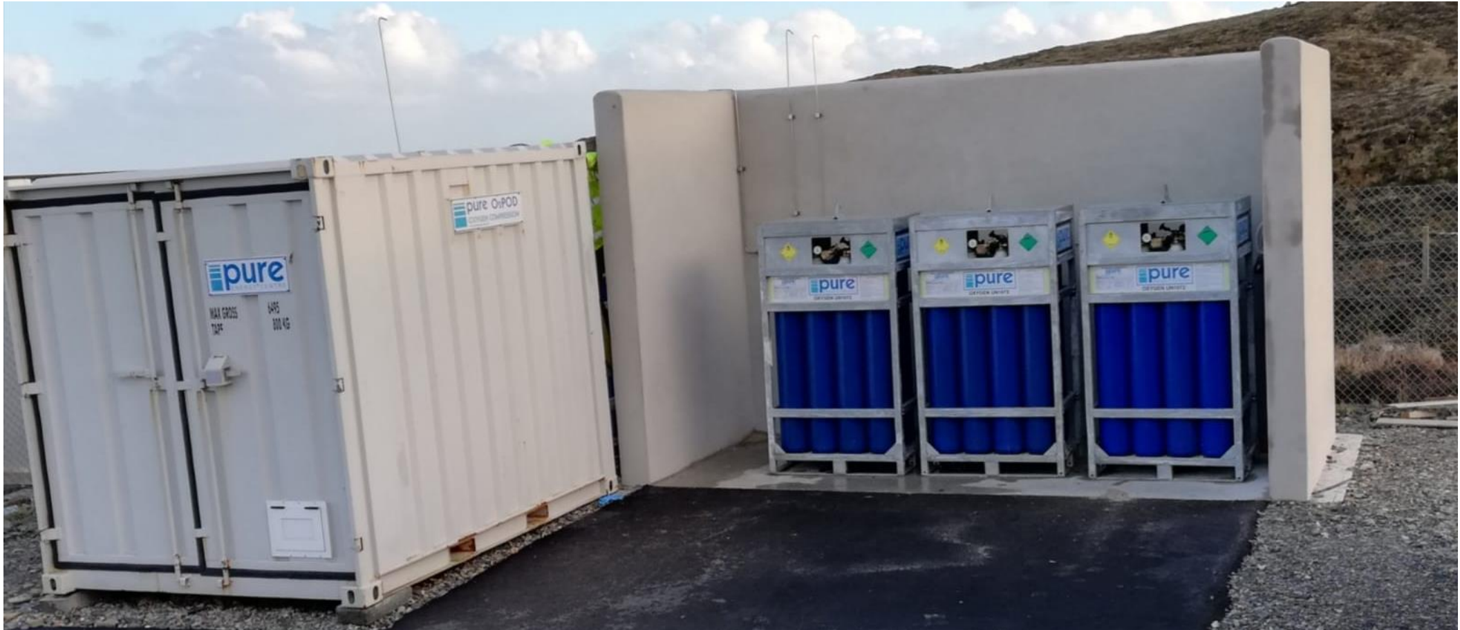
The Oxygen filling station
