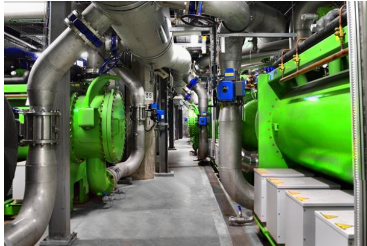
Figure 8: The cool production and storage facility of the Opéra, district cooling of Paris (Source: Climespace)
