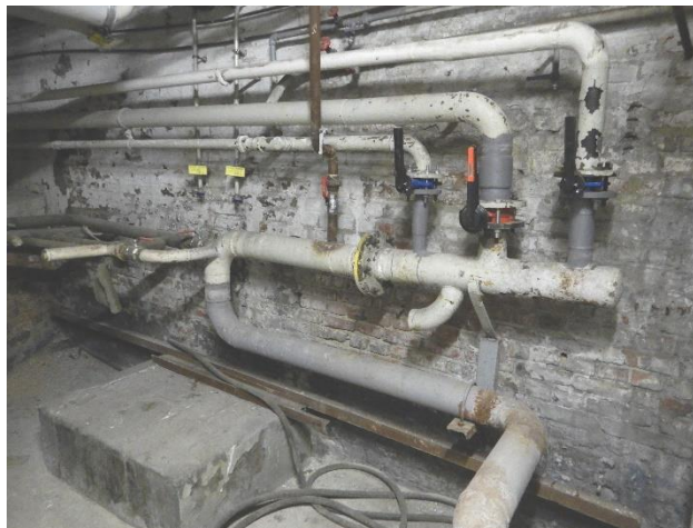
Figure 12: Absence of insulation on the secondary network's pipes
