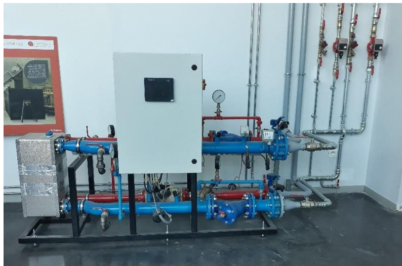
Figure 10: Demonstration copy of a substation, District Heating of Roubaix, France
